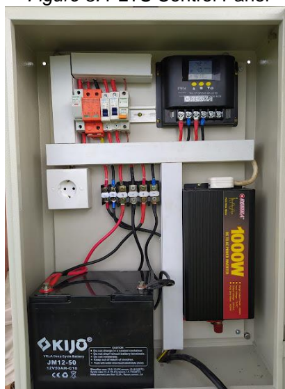
Figure 3. PLTS Control Panel
