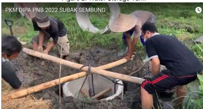
Figure 2. Water Storage Tank
