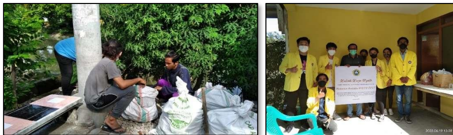
Figure 10. From Left: Cleaning and transporting remnants of construction materials; Right: handover event with RT 04 Wisma Permai
